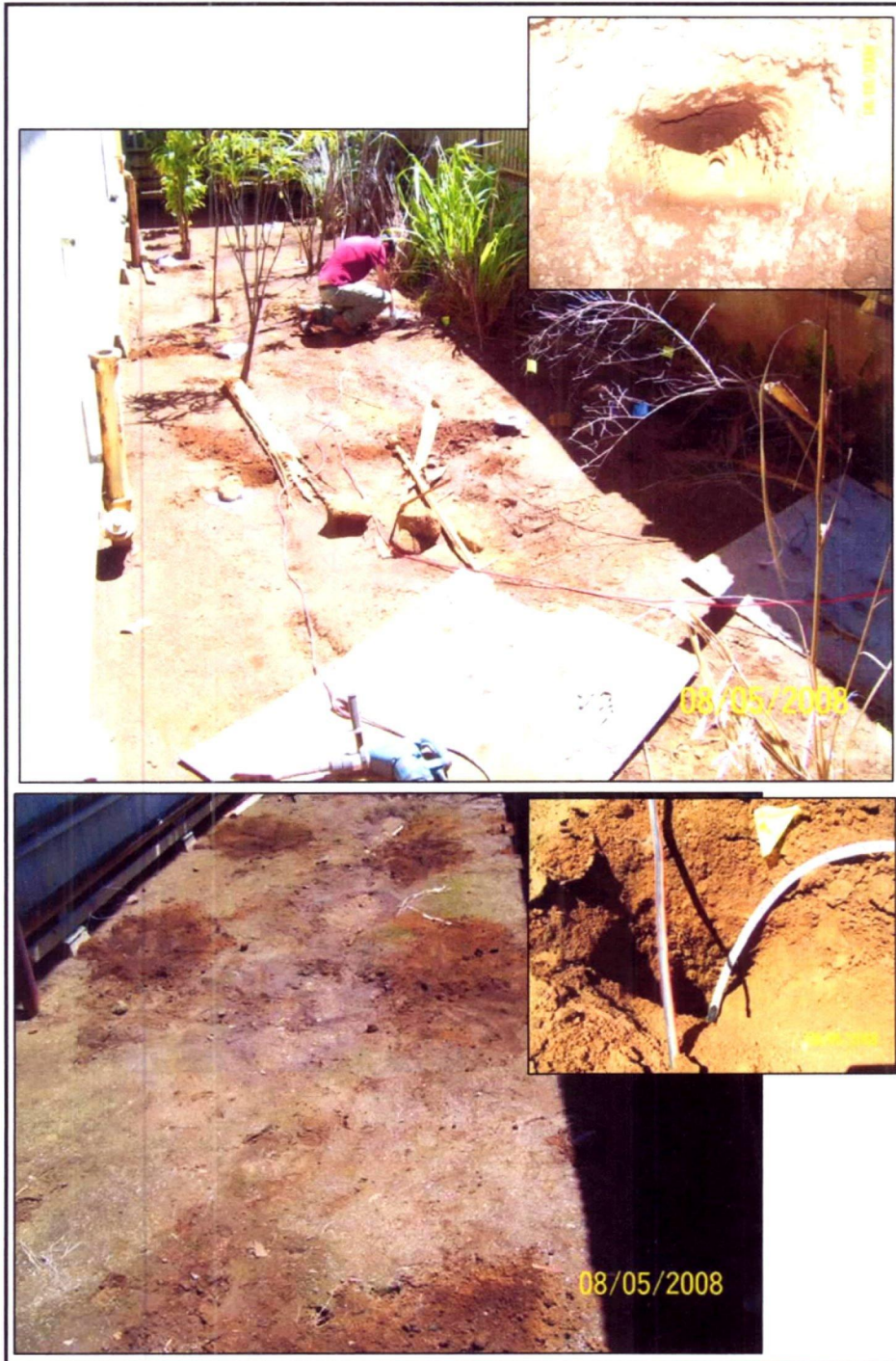
Subsurface characterization study to determine the extent of lead contamination in the open area between the gym and the south and north annexes using an XRF meter. Samples were taken at different locations and depths (6, 12, 18, and 24 inches bgs).
