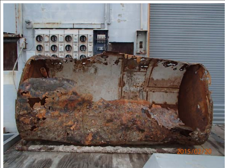
Photograph 10: 500-gallon UST in poor condition.
