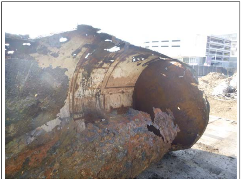
Photograph 5: Bottom of 500-gallon UST following removal - completely corroded.
