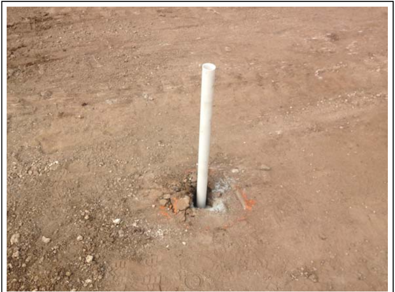
Photograph 13: Temporary monitoring well MW2.
