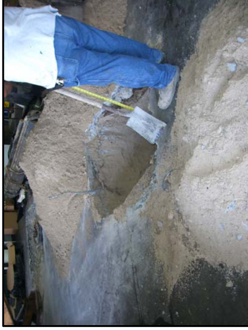
Photo 4. M. Nakai personnel backfilling the H2 excavation. Note no staining was observed.
