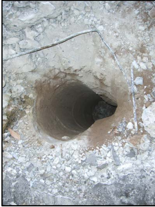
Photo 3. The H1 excavation after the removal of the hoist. Note no staining was observed.
