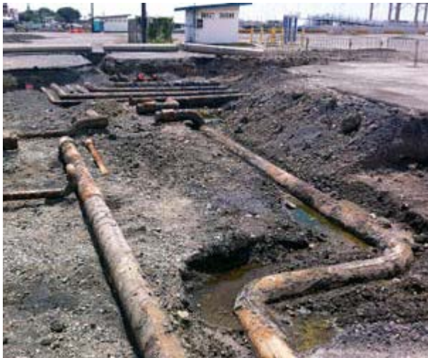
Exposed abandoned pipelines in the harbor area.
