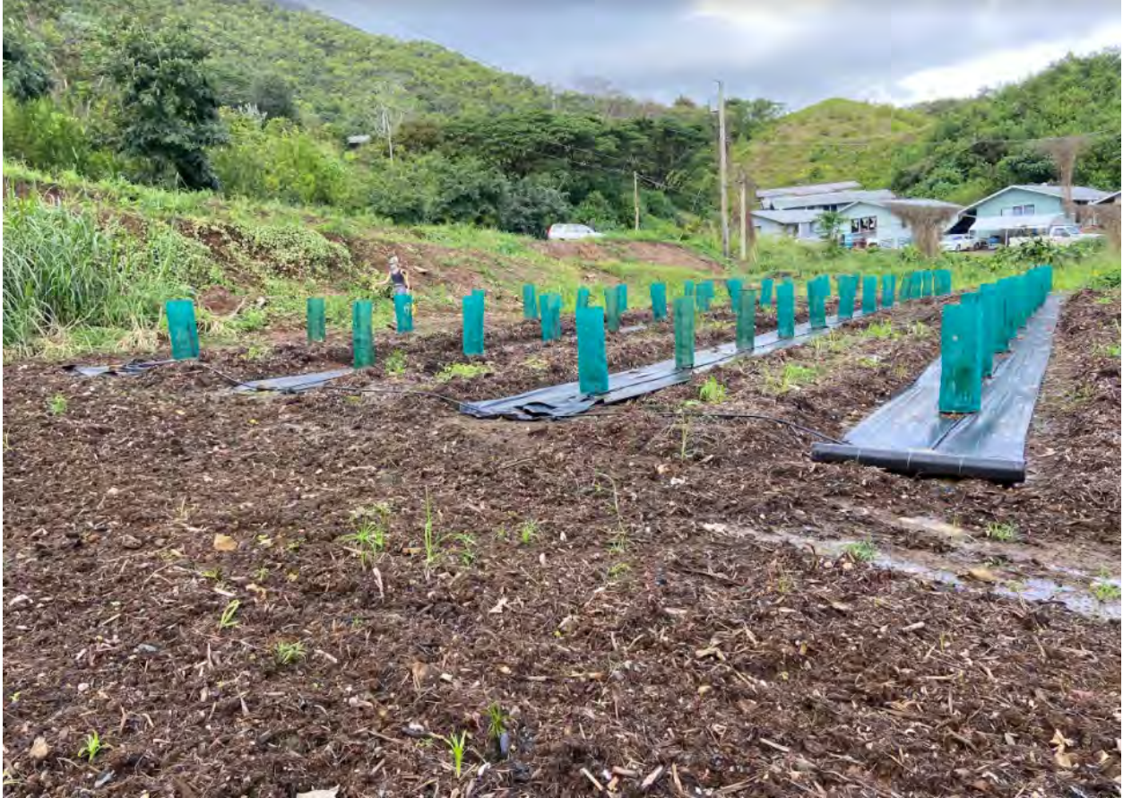
Image above: The slope above the cacao orchard will be stabilized through a critical area planting. This additional conservation practice will slow and filter surface waters that runoff from the mountain and prevent the slope from eroding and sediment from entering the waterways.
