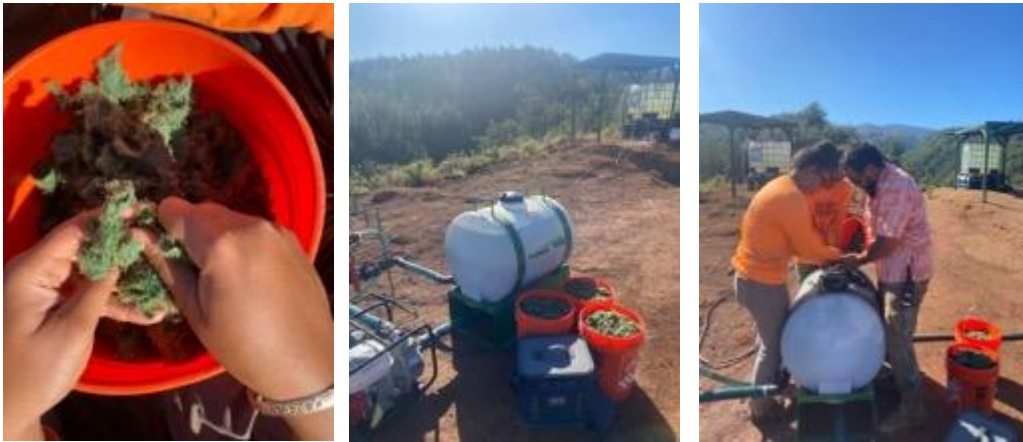
(Pictured from left to right): Fiber Tackifier prepared for hydroseeding; the Turbo Turf Hydroseeder and equipment assembled on site; PKW field crew adding the hydroseeding components to the machine.
